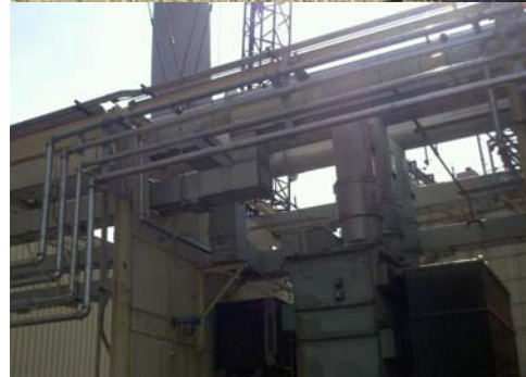
F.E. Moran removed all of the existing piping and installed a comprehensive deluge system to protect the facility's transformers
