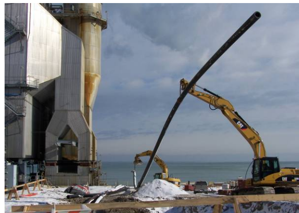
Installing and underground system requires knowledge and expertise; the Oak Creek Power Plant installation involved a complex excavation to achieve the proper installation technique.
