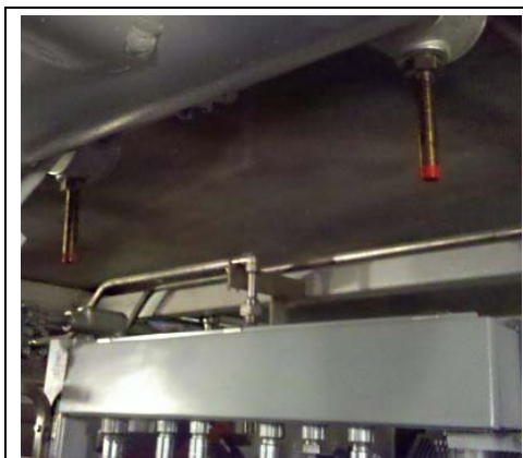
When the turbine manufacturer's drawings for the CO2 system did not meet the AHJ's requirements, F.E. Moran's designers and technicians immediately traveled on-site to modify the drawings and hand-deliver them to the AHJ for approval
