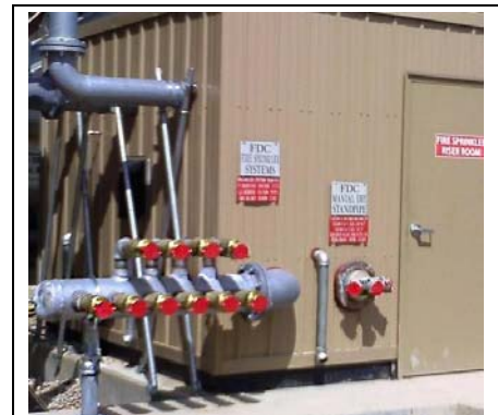
F.E. Moran used innovative design and installation techniques to satisfy the requirements of both the AHJ and insurance provider
