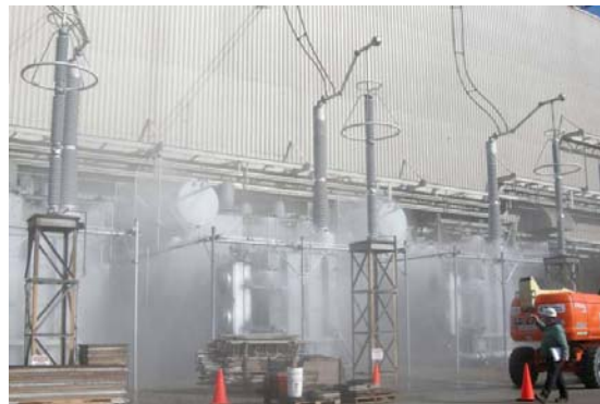
Developing an ongoing inspection, testing and maintenance regimen helps maximize the deluge system's life cycle.
